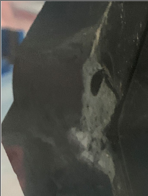
2 Medium damage: significant breakage of material or several small areas where material has been damaged revealing loose asbestos fibres (Plug-in board)
