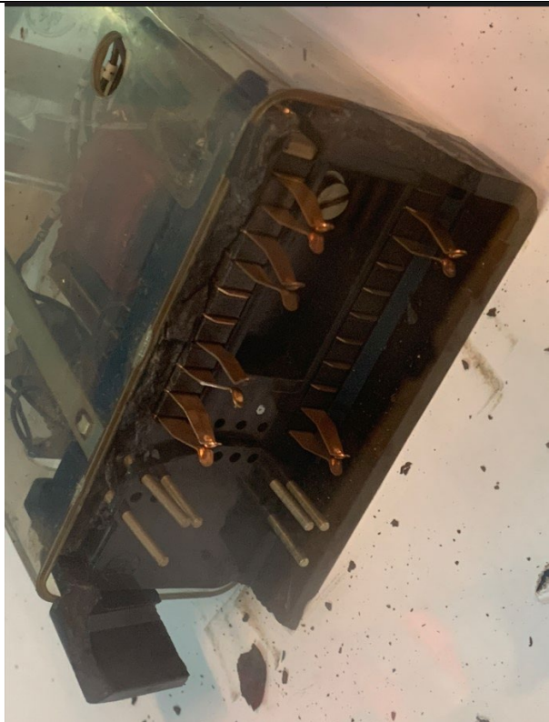
3 High damage or delaminated materials and thermal insulations. Visible asbestos debris
