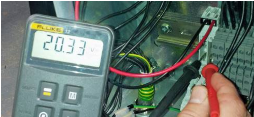
Figure 5 – Solar Panel Voltage Measurement
