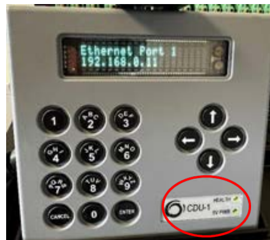
Figure 3 – Health & Power LEDs on CDU-1
