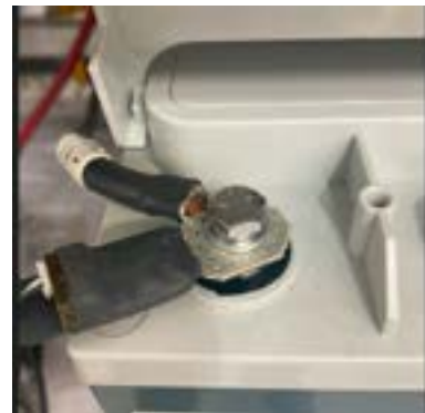
Figure 2 – Battery Terminal with Thermal Probe Fitted
