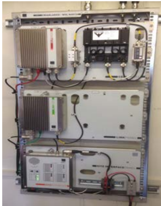
Figure 1 – Base Station Radio Modules
