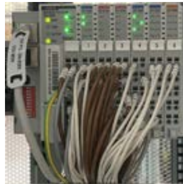
Figure 2 - Six RGTi ST Modules fitted to TCP-IP Router
