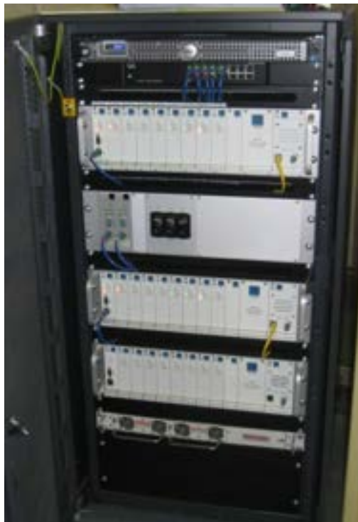
Figure 1 – RETB System Control Radio Rack
